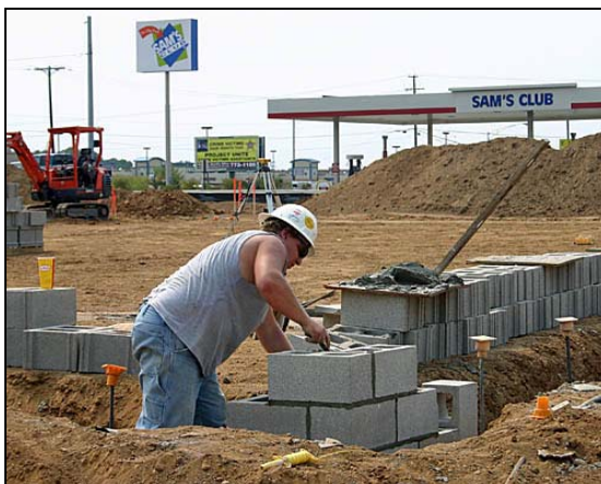
Block is laid for a multi-tenant building in front of Sam's Club on North Bridge Street.
