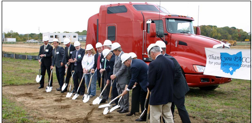
Ground is broken for the new PACCAR Medical Education Center on the campus of the Adena Health System in front of the present regional medical center and doctors office building.
